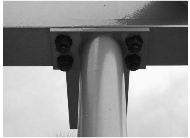
Figure 6-8. Column Connection: Base plate (bracing column) Girder B4 / Column C3 / Girder B8
