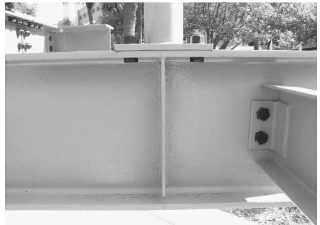
Figure 6-9. Column Connection: Base Plate (bracing column) Girder B4 / Column C3 / Girder B8
