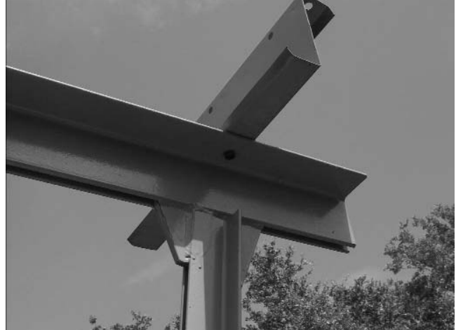
Figure 7-12. Misc. Connection: Z Purlin. Truss B7 / Purlin B9.
